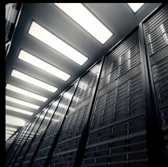
Data Centre and Infrastructure
